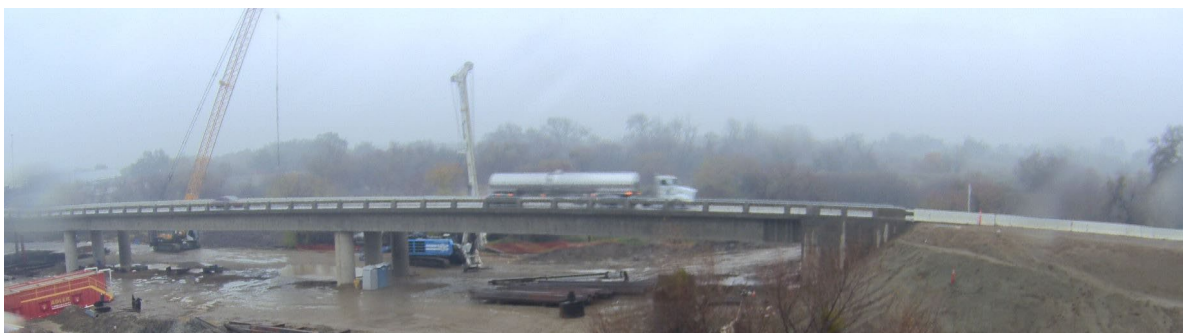
Photo of the new bridge structure looking from the north side of the new bridge.
