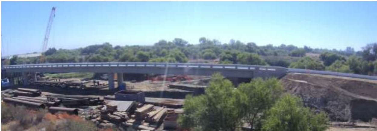
Photo of the new bridge structure looking from the north side of the new bridge.
